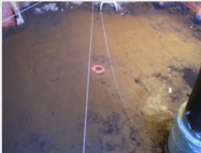
Interior surface compaction complete, ready for form work and pier footing pour
