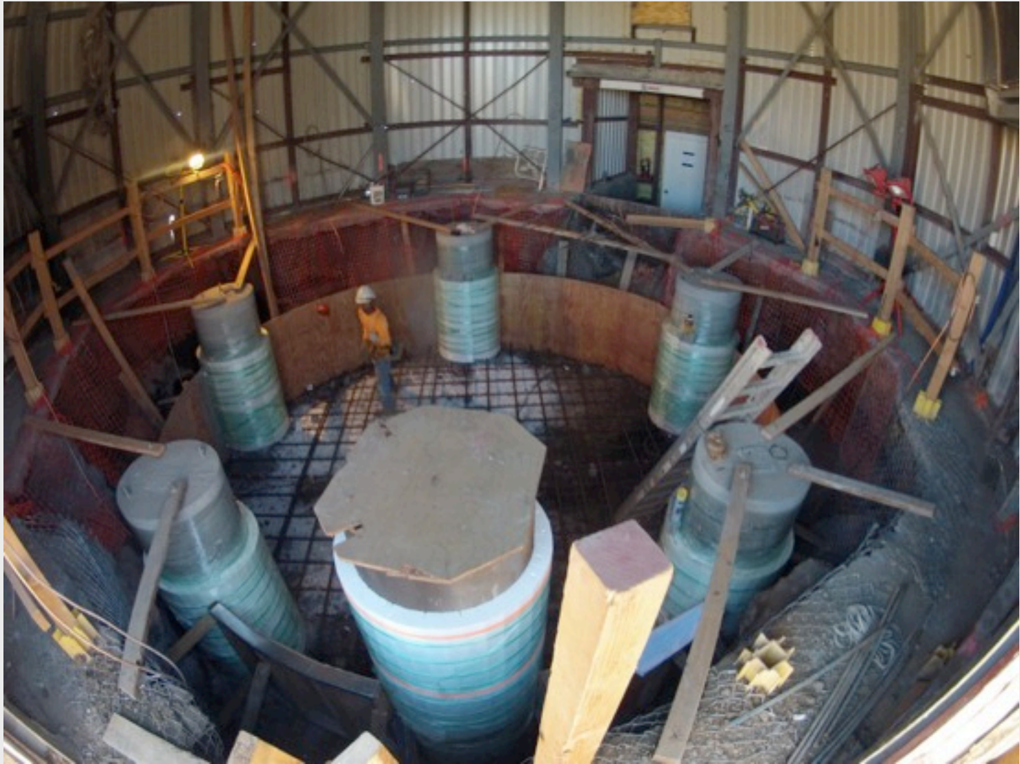
The pier footing rebar installation is shown from the tramway door (26 Dec 2012).
